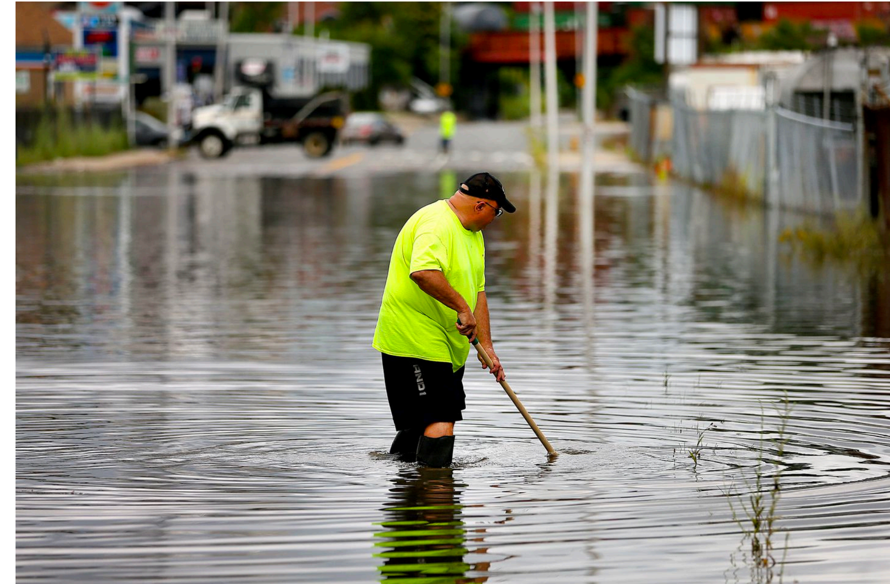
A Worcester DPW worker looked to unclog a storm drain on Southbridge Street in Worcester. JOHN TLUMACKI/GLOBE STAFF
